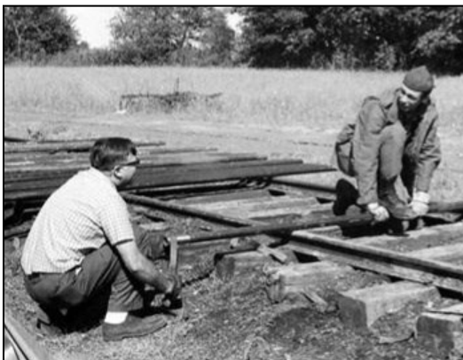
Above: Dick Stair (left) and Don are polishing the ends of flues for No. 1 boiler. Ted Lemen photo
