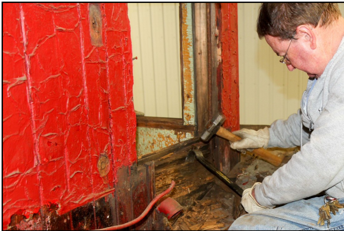
Dennis Sloan is in the process of removing rotted wood from the plow body.
