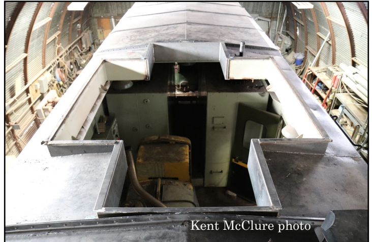
New roof hatch opening in CN15421. Width is as-built. We have extended the length of the opening to allow the new genset to drop straight in.
