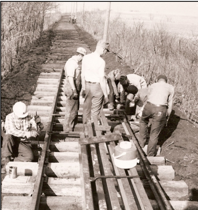
Hank (center; standing) is overseeing the laying of the rail on the “Hill” of the former IT main line .
