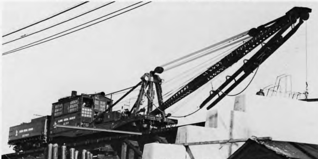
IC X17 STEAM PILE DRIVER. PHOTO BY WILLIAM A. RAIA. Shown during bridge rebuilding at Riverdale, IL in November, 1970. Retired from roster in 1990.
